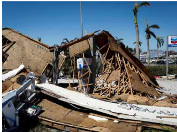
A destroyed gas station is seen after Hurricane Ian caused widespread destruction in Fort Myers, Florida
