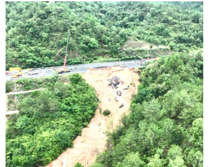
An aerial photograph published by state broadcaster CCTV showed wrecked vehicles lying in a deep muddy pit where the highway once ran.
