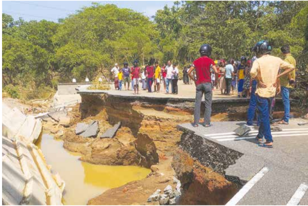
People gather around the Deduru Oya Bridge, which collapsed after floods in Kurunegala AFP | Colombo, Sri Lanka
