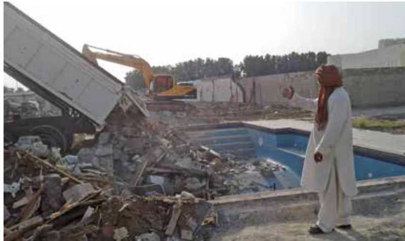
The swimming pool which was demolished by Southern Area Municipality in Dar Kulaib village near Hamad Town
