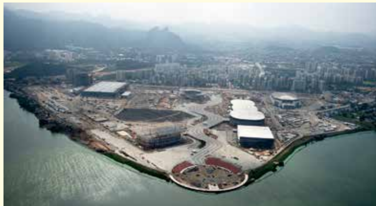
The Rio Olympic stadiums under construction from a metropolitan area of some 12 million people, into Guanabara Bay as a whole.
